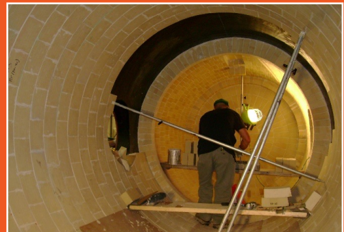
A worker at KMT workshop lining the tower with DURO™ Acid-Resistant Bricks and chemical-resistant mortars.
